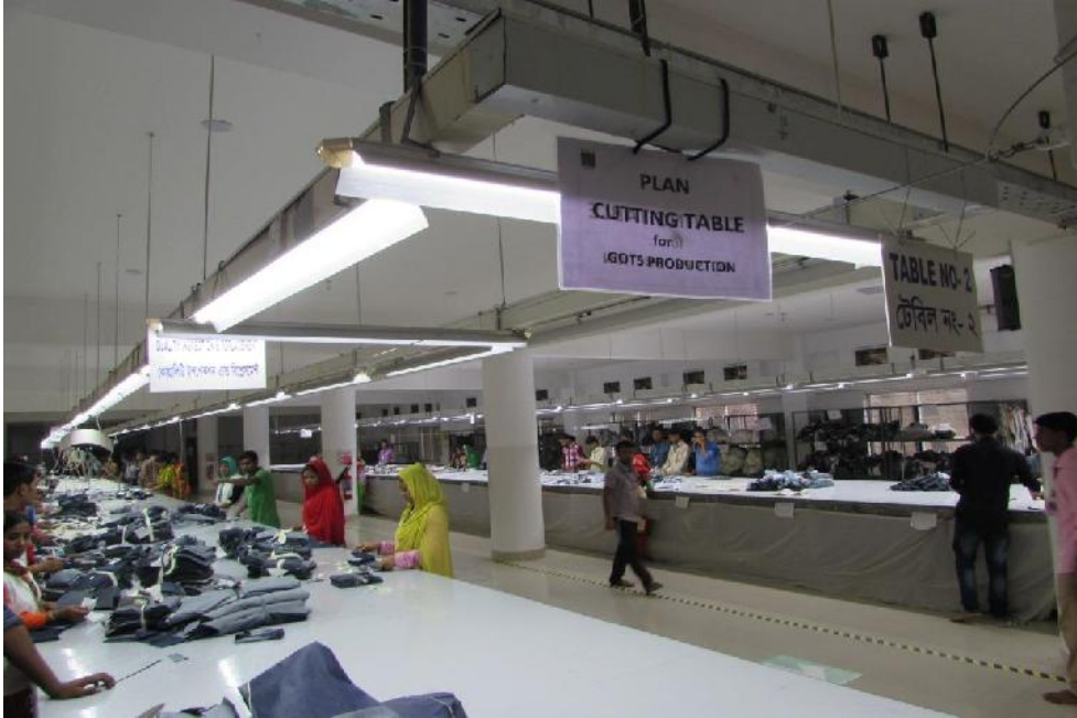
Figure 3: Electrical Installation on the factory floor.
